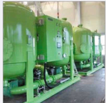
SAMSUNG TECHWIN AIR DRYER
