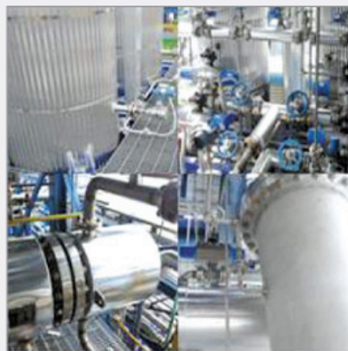
ISU CHEMICAL IPA DRYER
