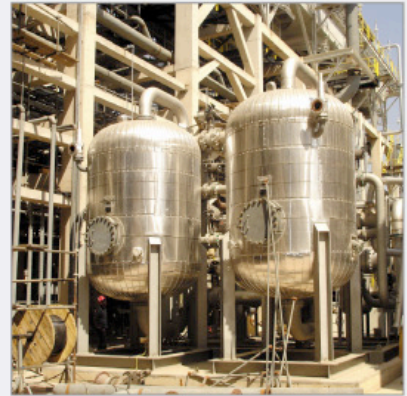
TUPRAS AIR DRYER
