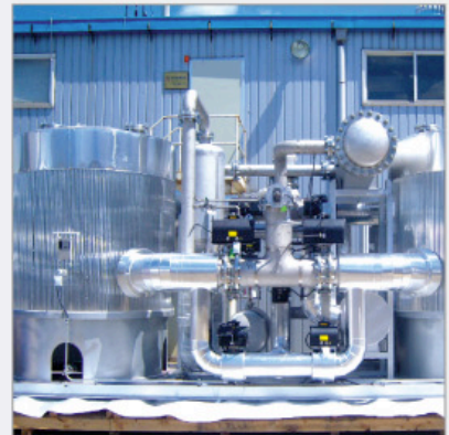
SK CHEMICAL N 2 DRYER
