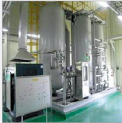
LG INNOTECH N 2 GENERATOR
